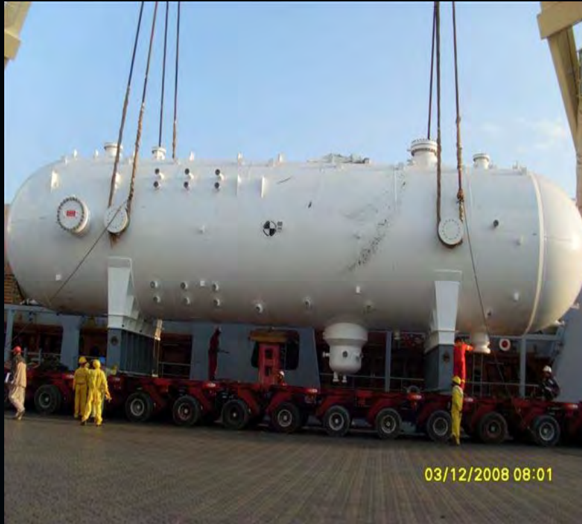
300 Ton HP separator being discharged at Abu Dhabi Port for onward movement by barge to Mussafah for Habshan OAG III Project
